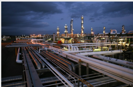
Maui production station, photo courtesy of Shell Todd Oil Services Limited
